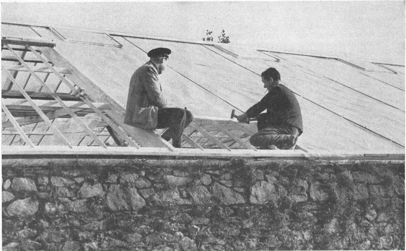
Covering the frame of a glasshouse in Gurnsey with five feet wide plastic. The plastic is being secured to the glazing bars with paper-tapes and a batten is applied to each joint. —Photo courtesy Dyes & Chemicals Ltd.
